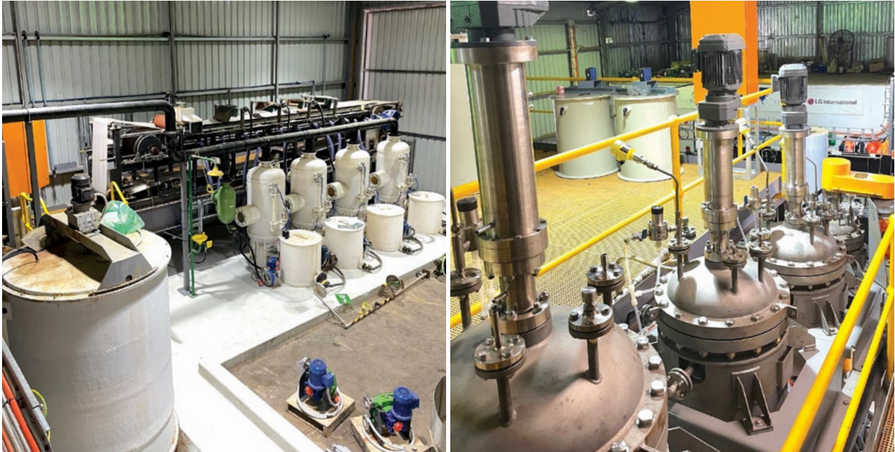
Figure 5 – Horizontal vacuum filter belt and Pressure oxidation leach circuit.
