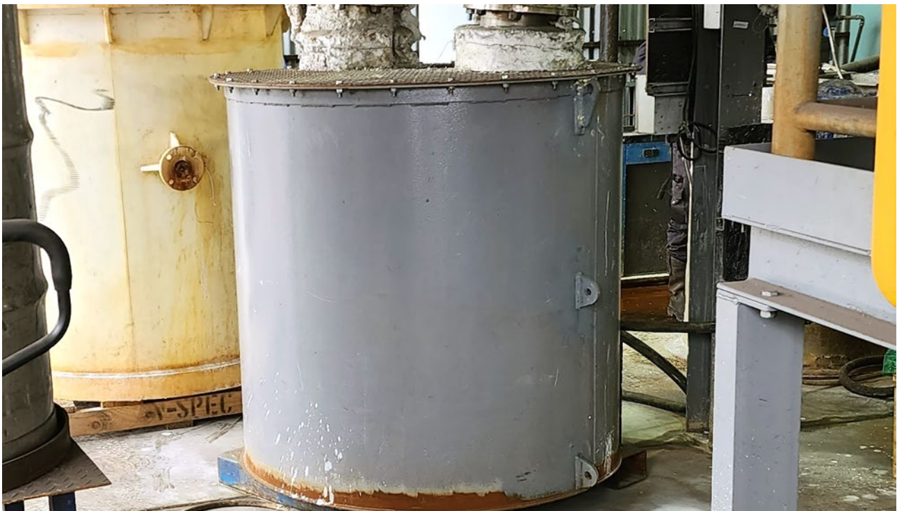
Figure 1 – Sulphur collection tank
