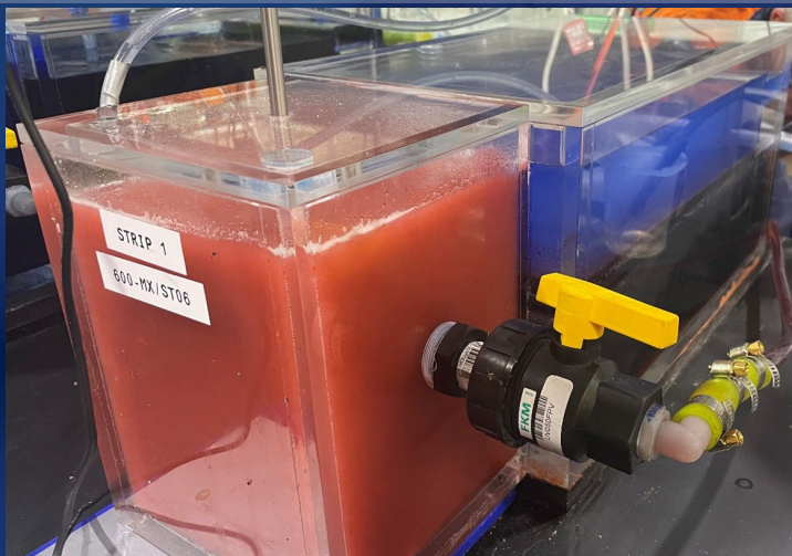
Cobalt Solvent Extraction Strip Cell
