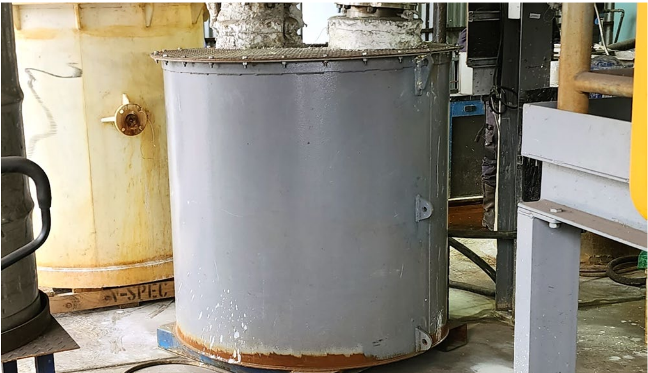
Figure 1 – Sulphur collection tank
