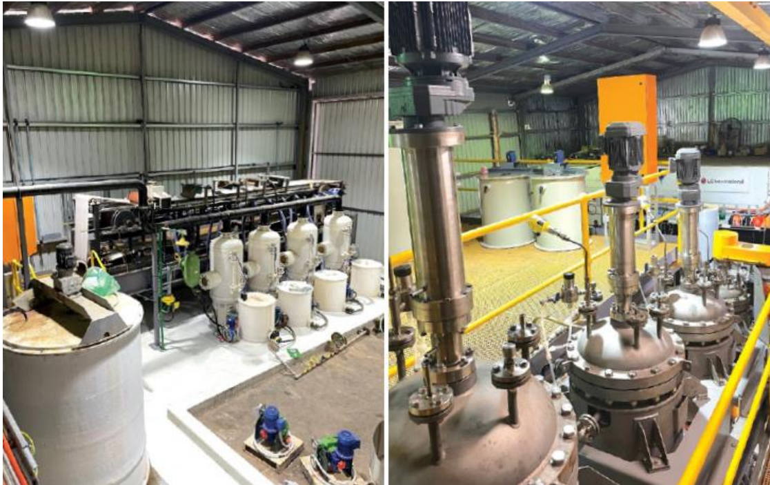
Horizontal vacuum filter belt & Pressure oxidation leach circuit
